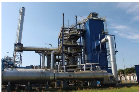
Waste heat boiler with the cleaning installation of EKOZUB Ltd. company working at Petrochemia Blachownia S.A.(Joint-stock company) -Kędzierzyn Koźle
