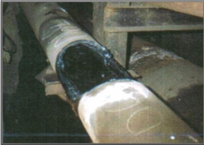
Inspection hole directly after the pump
