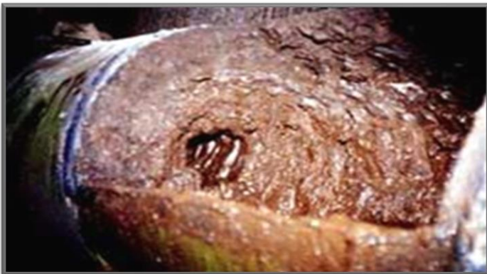
Contaminated pipe in 90% cross-section
