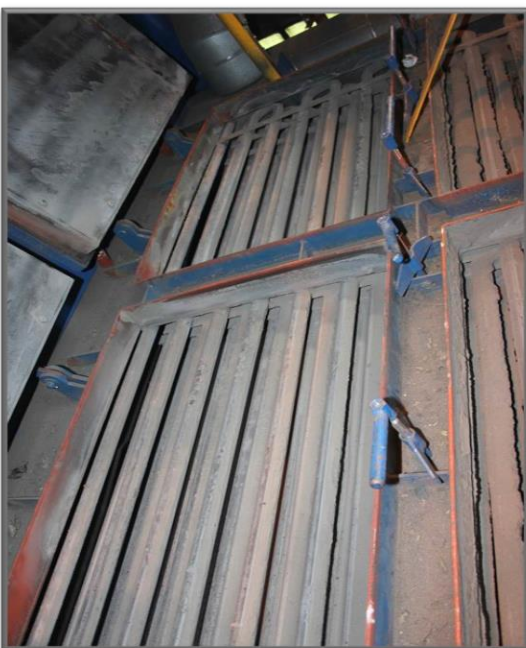
Additional boiler economiser WR-5 in MPEC Sp. z o.o. in Piekary Śląskie
