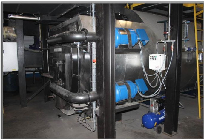
Incinerator medical waste in Konin
