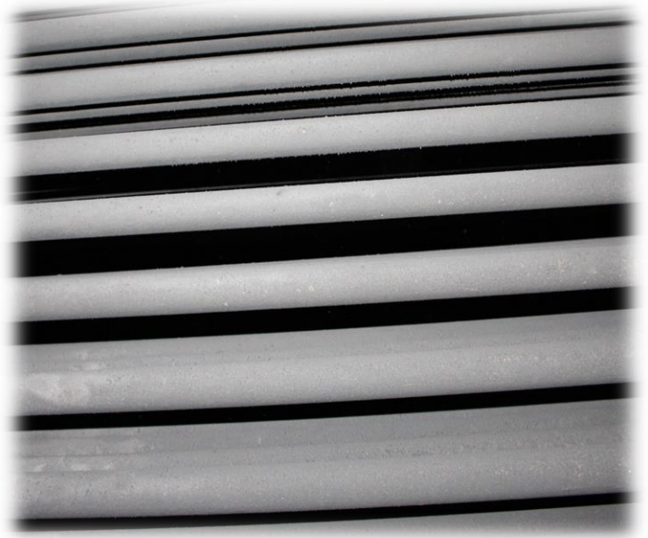
Water heater pipes without visible deposits, cleaned by a shockwave
